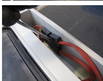
Fig. 37: Disconnecting the electrical plug connection
